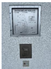
Fire alarm panel
