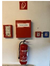
Fire brigade control panel/fire brigade plans
